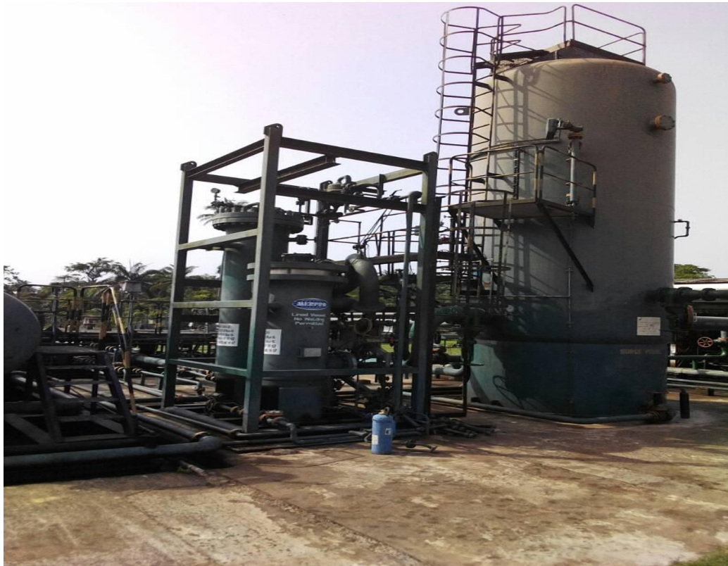
Plate 2. Surge Vessel Source: Author's field work, 2020
