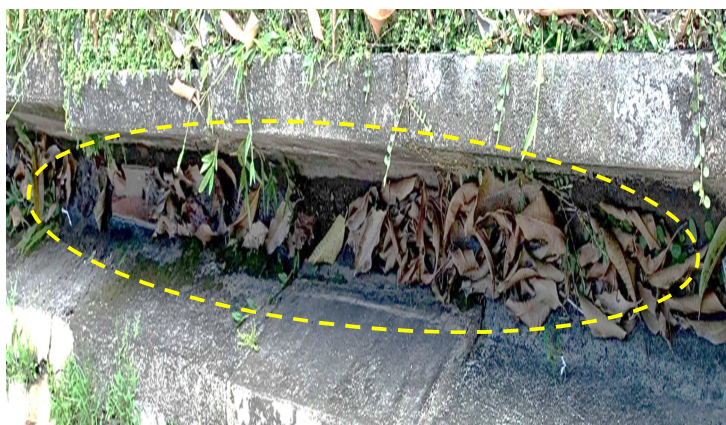
Fig. 8. Accumulation of leaves inside the drain
